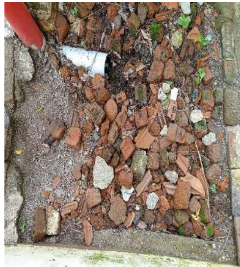
RAIN WATER HARVESTING PIT
