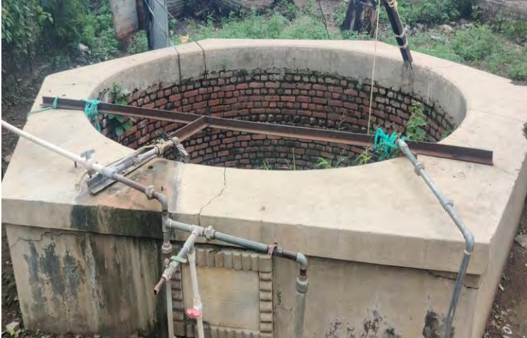
WATER WELL WITH PIPE
