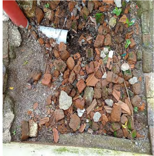
RAIN WATER HARVESTING PIT
