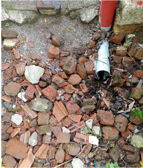
RAIN WATER HARVESTING PIT
